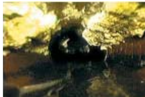
Actual photo taken by remote controlled camera, showing grease buildup in a sewer pipe.
